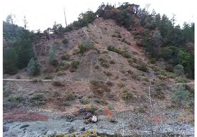
Figure 2.4.2-3 Landslide Undercutting the Rail Corridor at MP 244
